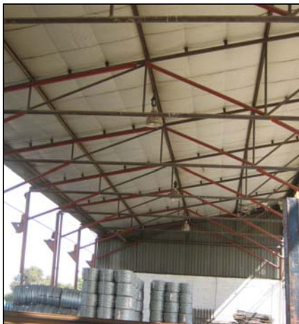
MAC STEEL STORE
